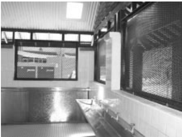
Interior of refurbished toilet. Wall sections have been cut away with dark coloured mesh instated.
