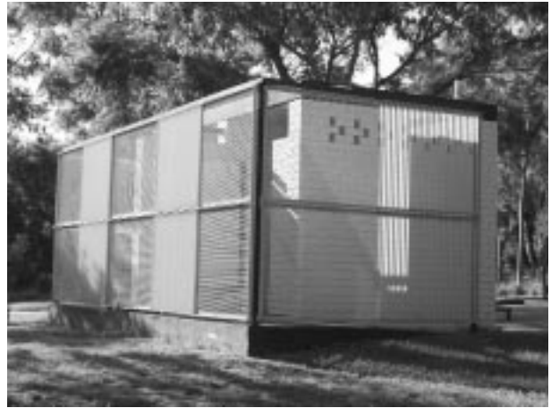
A major toilet redevelopment - external walls have been removed, and replaced with grills.
