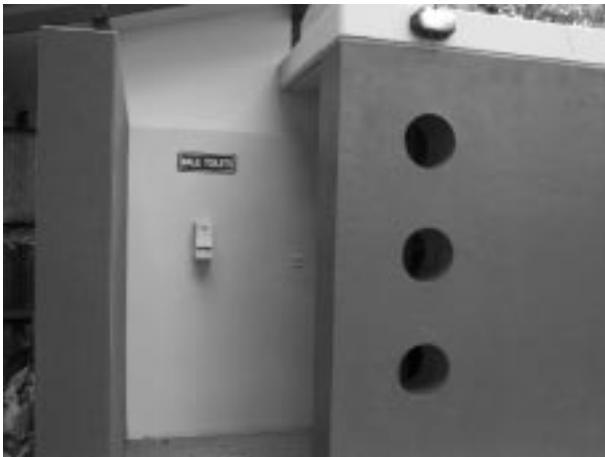
A section of wall has been removed (foreground) and holes have introduced.
