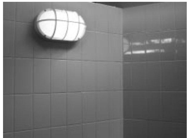
Lighting needs to be high mounted and vandal resistant. In this case, light coloured tiles assist with reflection.
