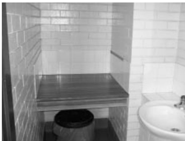
A basic parents room - small secure bench, opportunity for waste disposal & wash basin.
